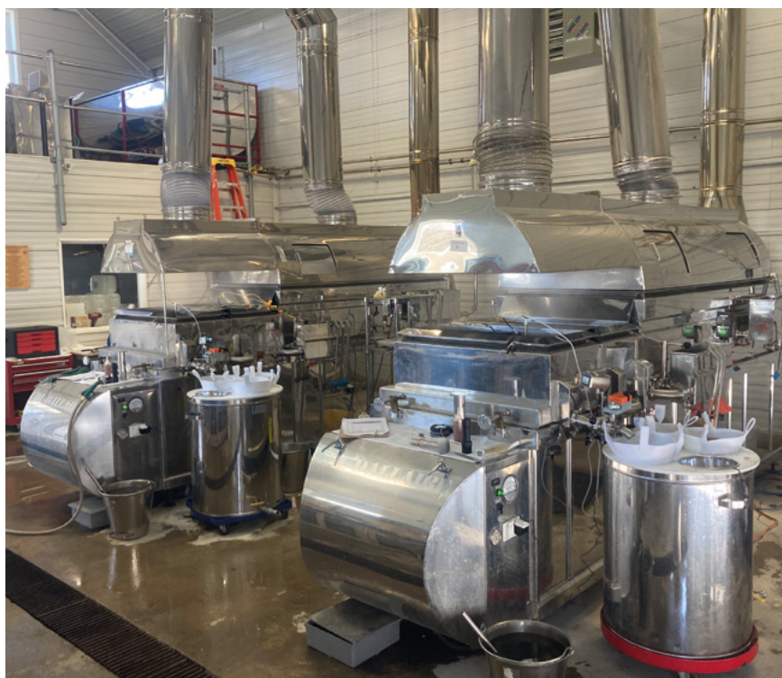
Fig. 2 – Maple Processing Research Facility at the University of Vermont Proctor Maple Research Center during an experiment processing pure red and sugar maple sap concentrated to 8%.
